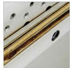
some rail profiles have dried lubricant residue present
